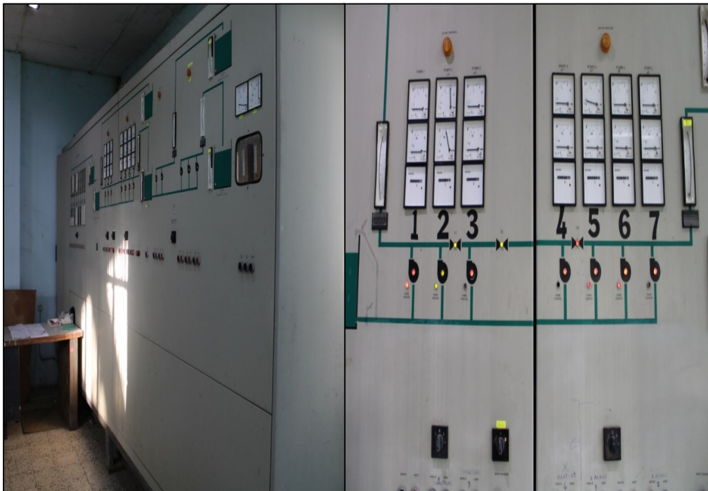
Figure 5. Armoire de commande (Photo Beldjerd).
